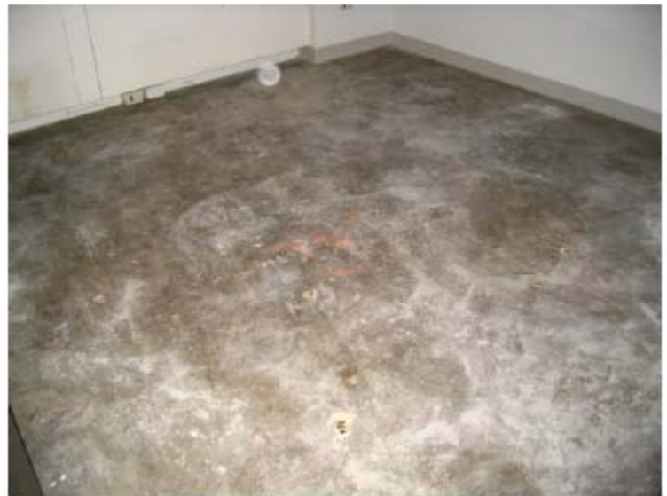
Figure 7: Floor 27 carpet water damage and visible mold (from Visual Mold Inspection Summary by TRC)
