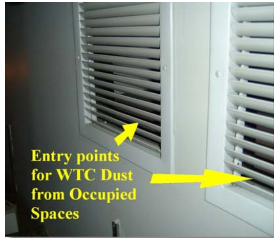
Figure 2. Walls with Louvers are Potential Pathways of Exposure to WTC Hazardous Substances. Reprinted from RJ Lee Group, TP-06 Contamination Report, 2003.
