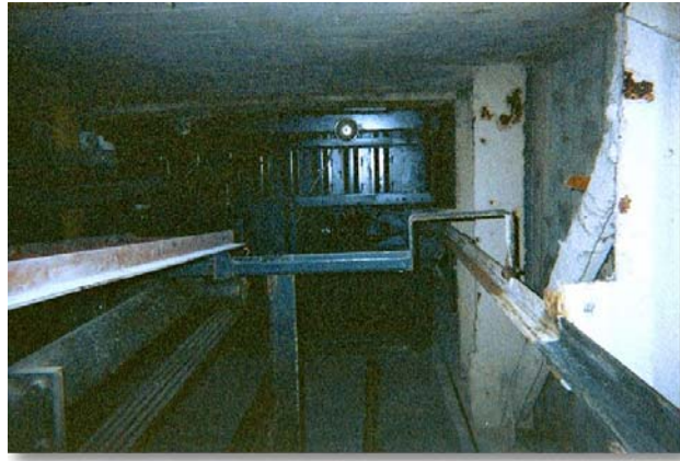
Figure 6. View of elevator shaft. Reprinted from RJ Lee Group, TP-12 Contamination Report, 2003.
