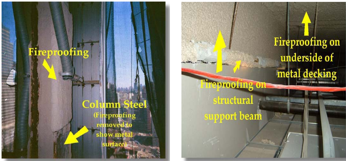
Figure 3. Fireproofing on column steel, structural beams and floor support. Reprinted from RJ Lee Group, TP-04 Contamination Report, 2003.
