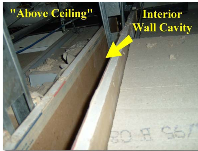
Figure 1. Interior “above ceiling” wall cavity. Reprinted from RJ Lee Group, TP-06 Contamination Report, 2003.
