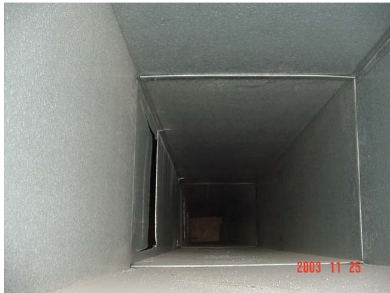
Figure 2. Low pressure ductwork.
