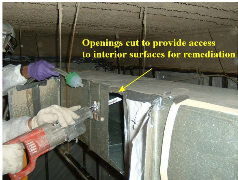
Figure 4. An opening is cut to gain access to the interior surfaces of low pressure ductwork.
