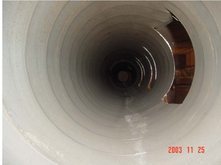
Figure 1. High pressure ductwork.
