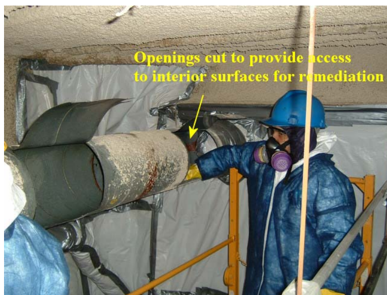
Figure 3. Access to interior surfaces of high pressure ductwork.
