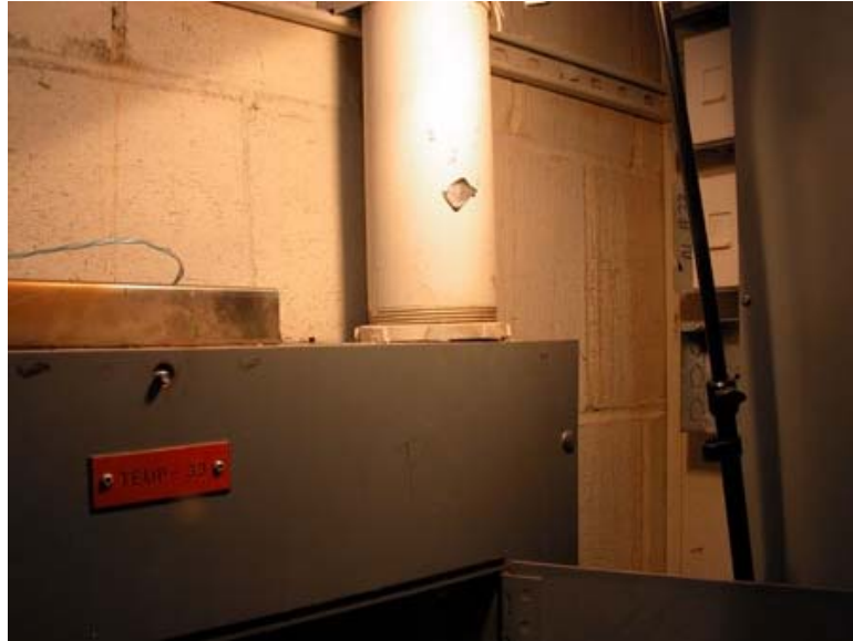
Figure 1. Beginning of Conduit Pathway on Floor 33.
