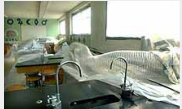
The News-Times/Wendy Carlson Clean air is filtered out of the chemistry rooms from a tube connected to a machine called a microtrap, which collects the air and sends it through its filters to remove asbestos particles.
